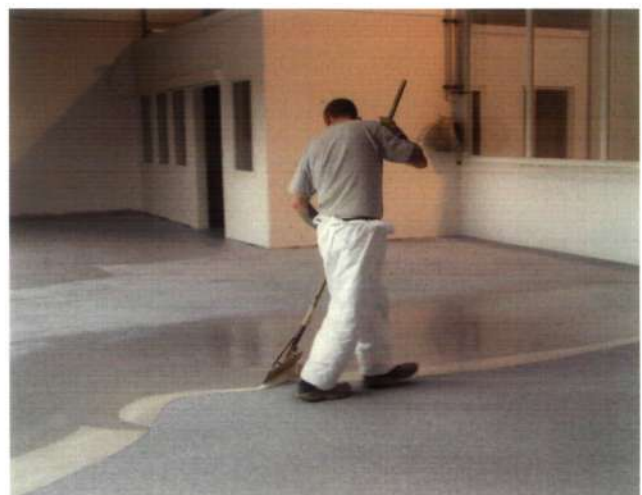
With the help of a long-handled spreader, an adequate safe working distance has been applied, reducing the likelihood of contact with the coating. It reduces the potential for back problems too.
