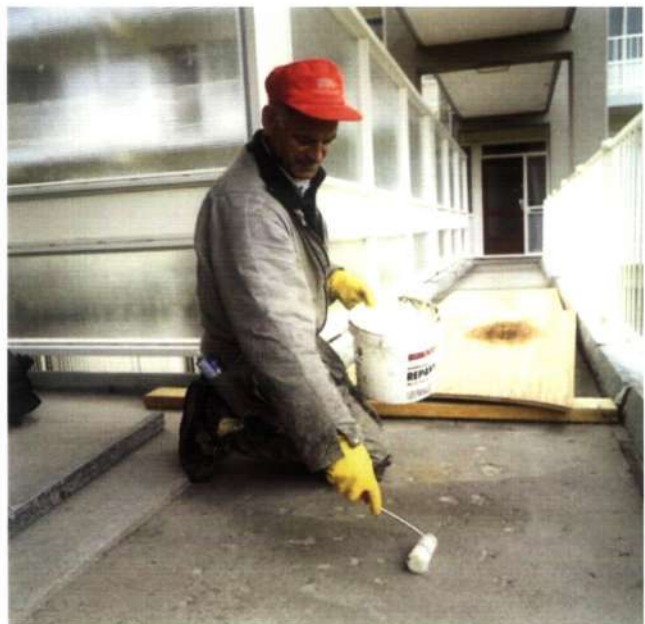
A floor coating being applied by a worker who is kneeling down and using a short-handled spreader.
